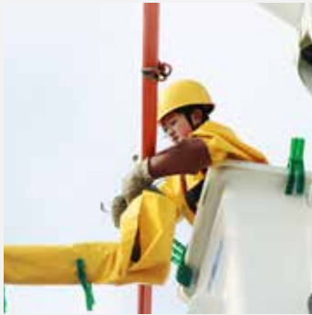
Women engineers working on high voltage electrical systems. © Chinese Society for Electrical Engineering
