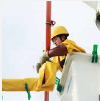
Women engineers working on high voltage electrical systems. © Chinese Society for Electrical Engineering
