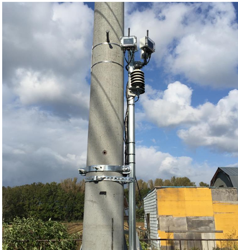
Figure 5.20. Sensor modules installed in the northernmost Japanese island Hokkaido.
