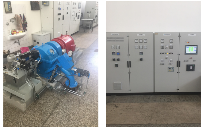
(a) HPP unit
