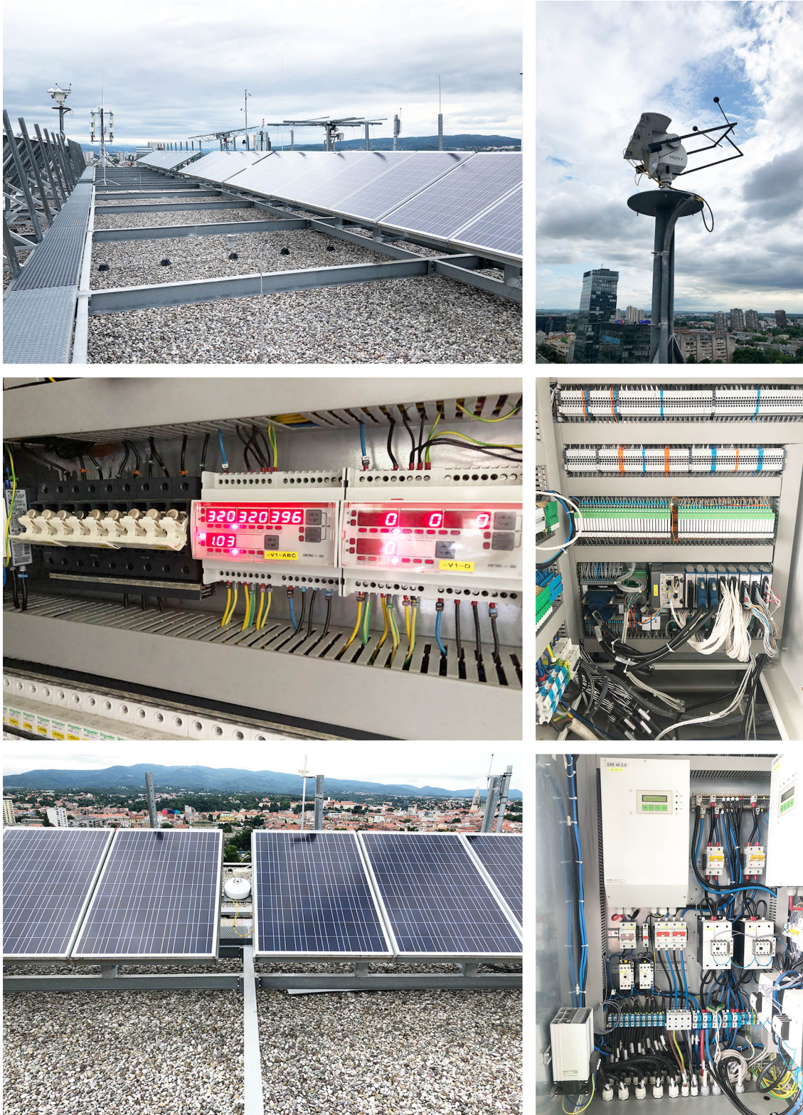
Figure 2.2: Equipment in LARES. From left to right, top to bottom: (i) PV arrays placed at fixed tilt angle to horizontal surface, (ii) Solys2 sun tracker with CHP1 pyrheliometer, two CMP11 pyranometers, and shading balls for diffuse solar irradiance, (iii) three-phase multimeters placed at solar inverter output, (iv) electrical cabinet with microgrid industrial controller and its peripheral, (v) pyranometer to measure solar irradiance incident with the PV array active surface, and (vi) electrical cabinet with microgrid power converters, contactors, automatic circuit breakers etc.
