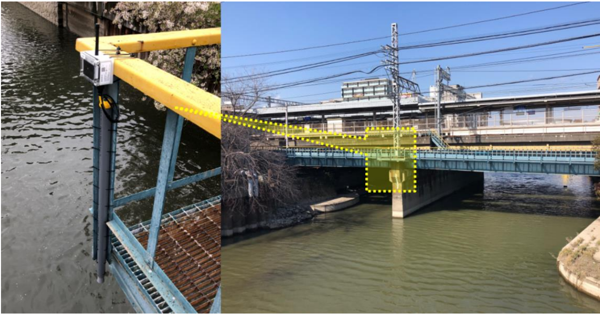
Figure 5.27. Ultrasonic sensor attached to a sensor module used for river water level monitoring.
