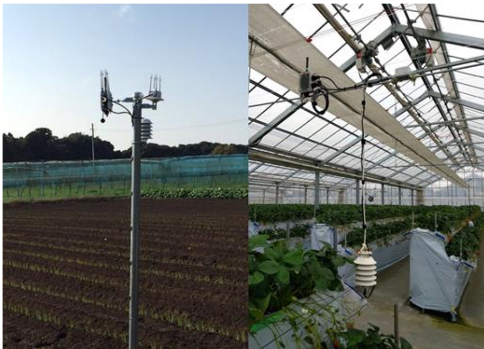
Figure 5.11. A sensor module with illuminance and ambient air temperature and humidity sensors attached, at the Chiba and Niigata test sites in Japan. Left is the outdoor installation in an onion field (Chiba) and on the right is the installation in a greenhouse used to grow strawberries (Niigata).
